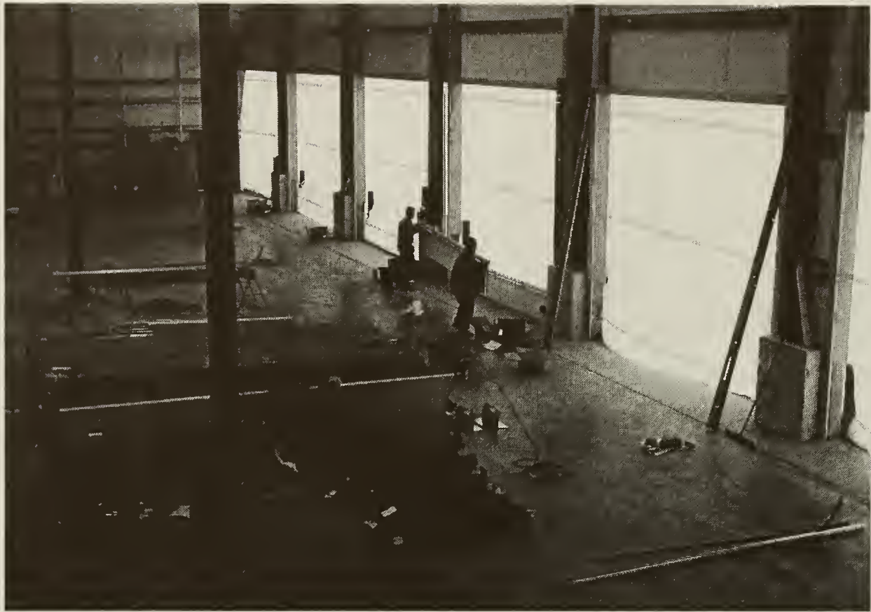
November 16, 2004. Installing the overhead doors by Twin State Door of Lebanon, NH.
